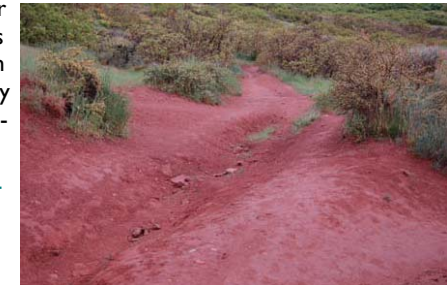
A portion of Skyline Trail showing serious erosion problems. Photograph courtesy of Jeff Porucznik.
